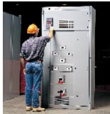
Digitrip OPTIM Trip Units can be easily programmed and monitored at the switchboard using the Breaker Interface Module. A hinged compartment houses the BIM and a 30 V Dc power supply for communications capability. For OPTIM 1050 Trip Units, a potential transformer module is supplied to provide voltage for power and energy monitoring.
